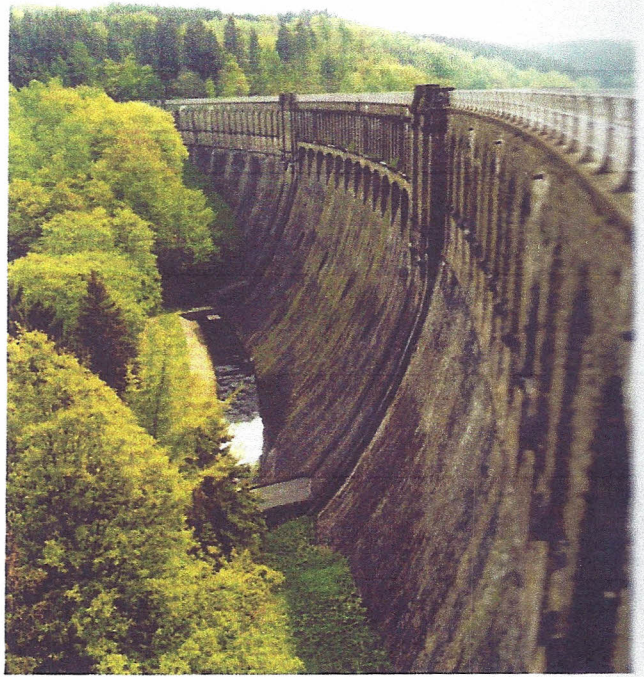
Above: Illustration showing the rehabilitation concept . Right: View of the 51m high Ennepe dam, which was built in 1904
